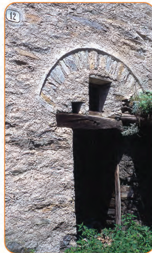
■ Entrance door with buttress. This kind of structure discharges the weight of the masonry above to the lateral supports.
